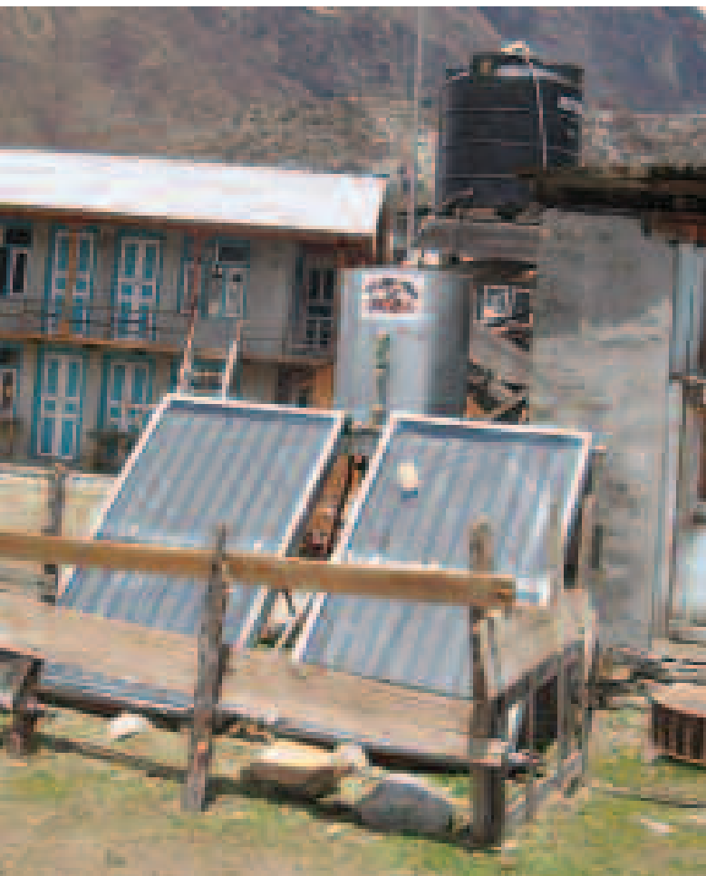
Solar water heating, Langtang, Nepal. Photo: Marianne Heredge.
