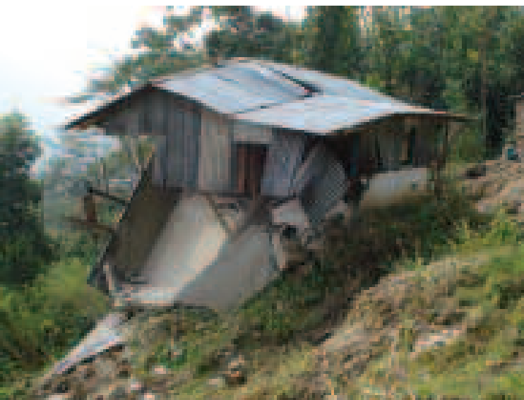
House destroyed in Harsing. Photo: MARG.
